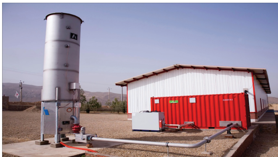
Figure 1: Shiraz biogas power plant with gas collection wells
